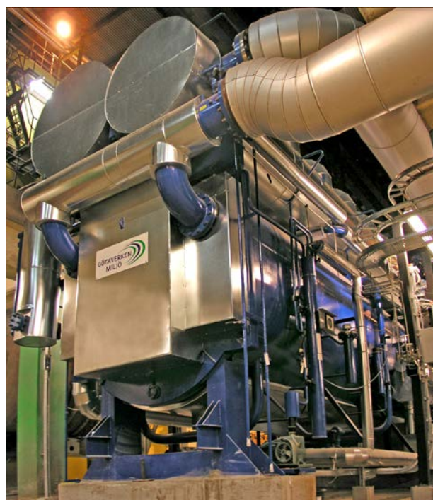
Absorption heat pump at Vestforbrænding, Denmark.
