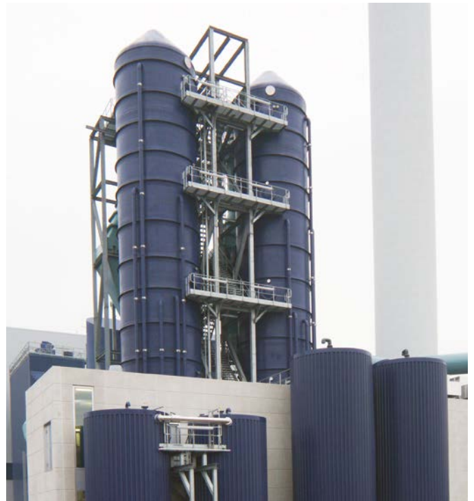
Condensing wet scrubbers at Maabjerg Energy Center, Denmark
